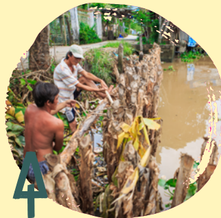
After receiving construction materials and technical training as part of the Foundation's ACCCRN work, local community members take flood prevention into their own hands, constructing several kilometers of erosion barriers along the riverside.
