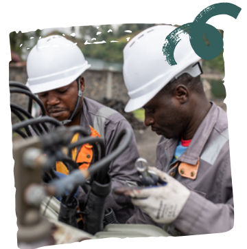
Two employees from Nuzu, supplier of the first Congolese solar mini-grid, work on the installation of new power lines in Goma, Democratic Republic of Congo. Global Energy Alliance for People and Planet.
